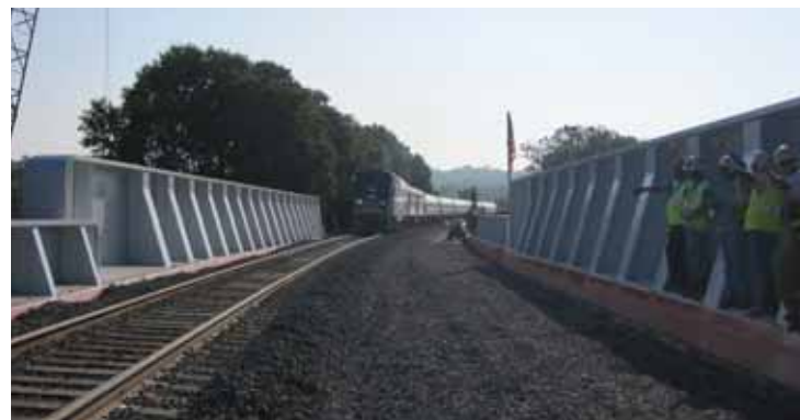
Crews cheer as the first train over the new Alexandria, VA, flyover—southbound Amtrak train 67—crosses on June 2, 2010. This bridge, jointly funded by Virginia and CSX, carries CSX’s main over NS’s.
